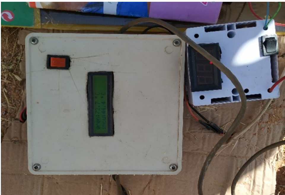
Figure 1: Temperature Control with Battery Bank.
