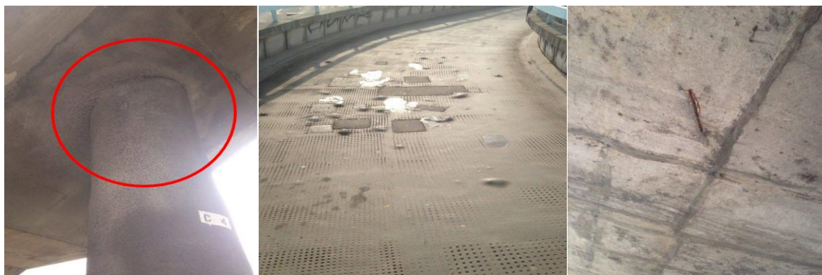
Figure 12: Defaults and cracks in Churchill Way flyover.
