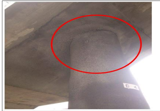
Figure 6: A portion of column C4 located under the stairs that have been repaired.
