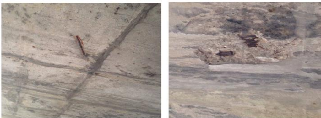
Figure 2: The underside of the Churchill Way flyover, rust coloured stain marks.
