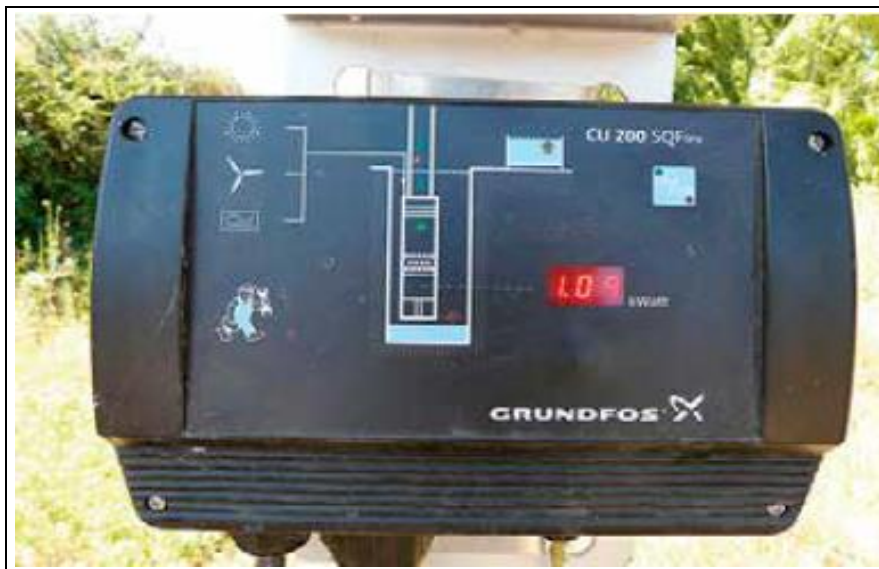
Figure 9: Solar pump controller and inverter [41].
